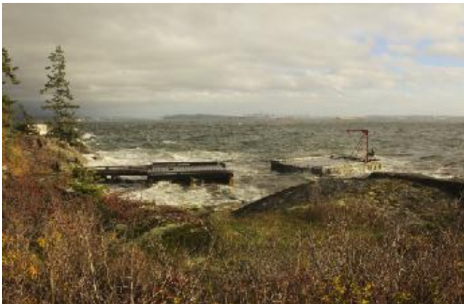
Point Atkinson wharf wrecked during winter storm, 2018.
